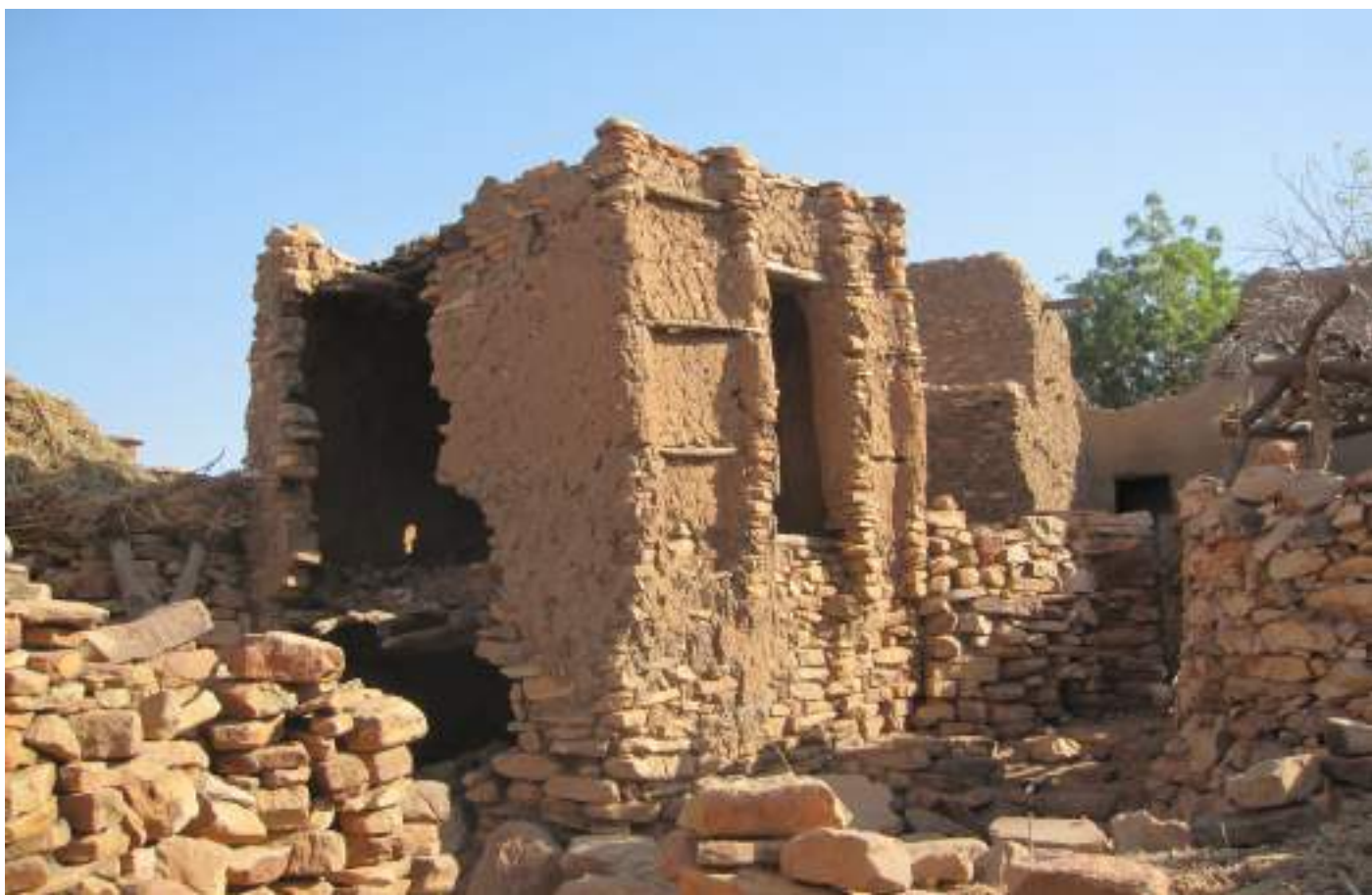
The start of collapsing
