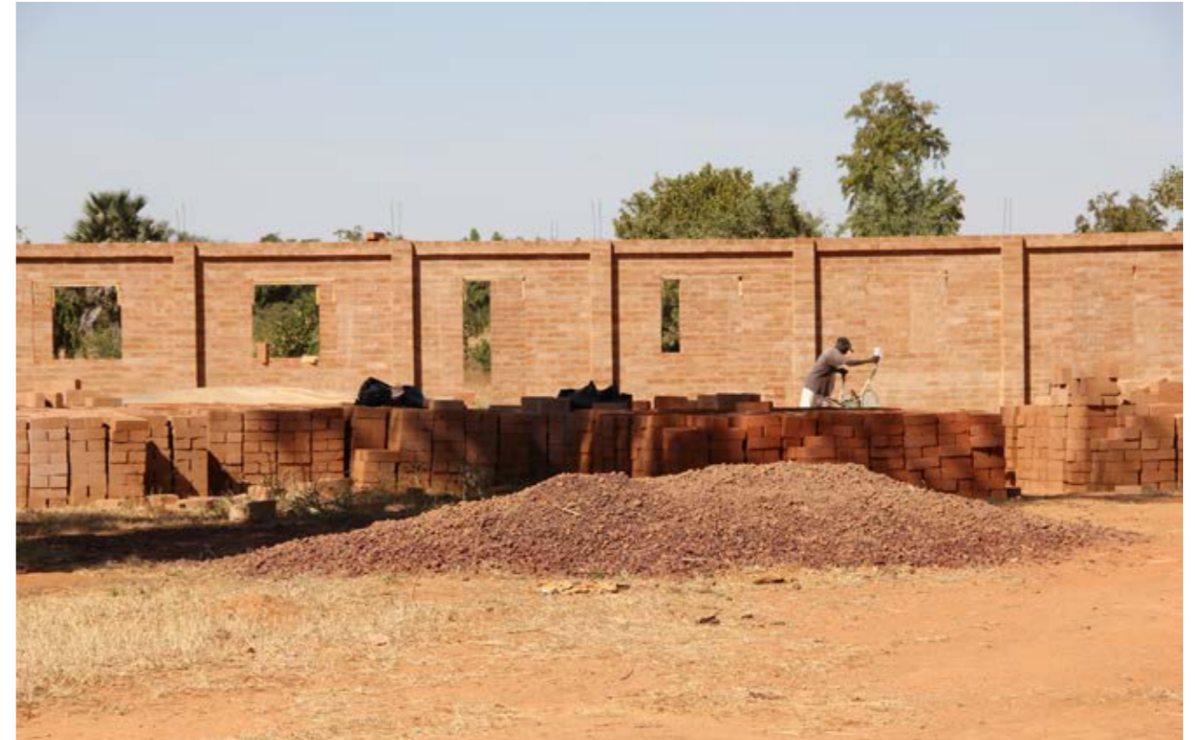
Left The earth block compressing machine is used on the construction site.
