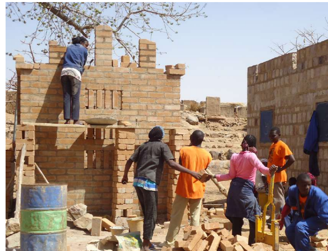
Internship of 8 students of the Technical School in Sévéré; the construction of the storage facility for onions
