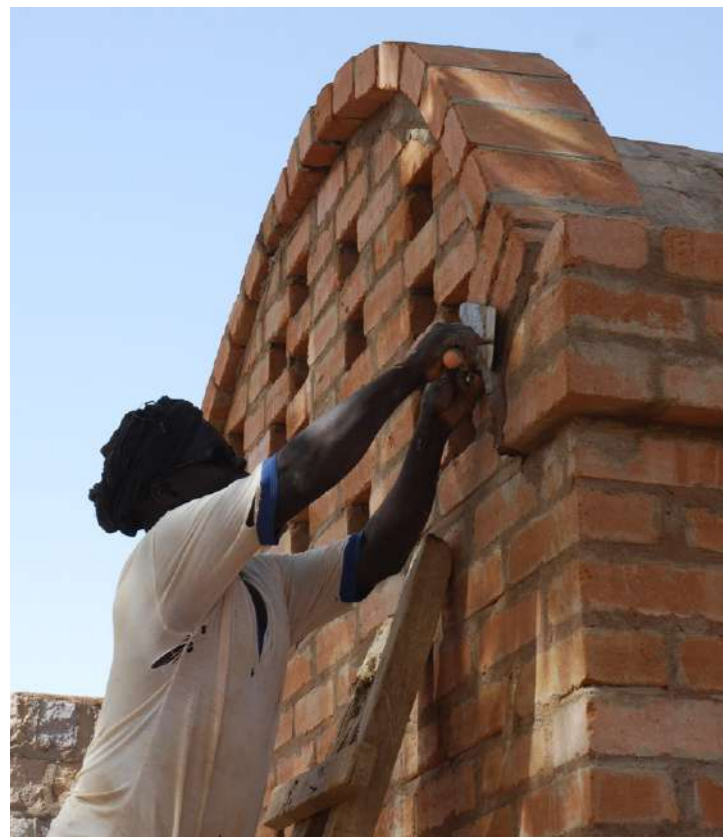
Internship of 8 students of the Technical School in Sévéré; the construction of the storage facility for onions
